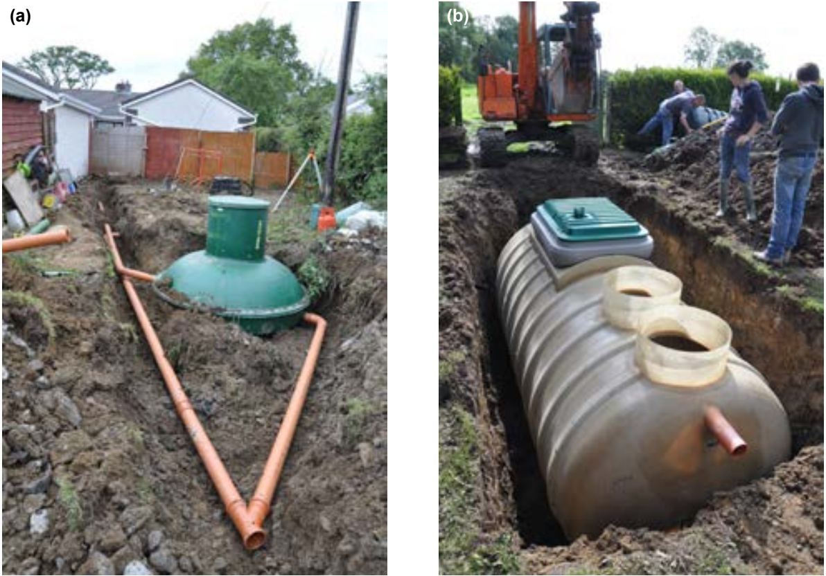
Figure 2.16. Packaged treatment plants: (a) extended aeration process at Site A and (b) media filter at Site B.
